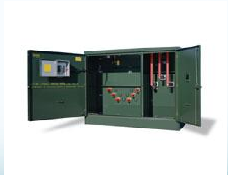
Figure 22 Pad Mounted Transformer
